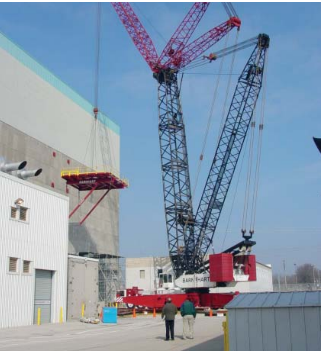
Left: A temporary platform was assembled on the exterior of the Quad Cities reactor building in anticipation of accepting a pair of new steam dryers that ultimately would be installed in the plant's boiling water reactors. After the platform was assembled, a hole was cut and a doorway placed in the building's side. (Photos, pp. 41-44: Barnhart Crane and Rigging)
